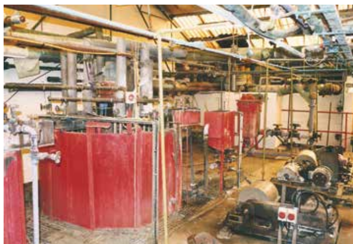
▲ Figure 1. Wastewater treatment is typically not given the same priority and attention as the primary process plant. Neglected plants may suffer from numerous issues.
